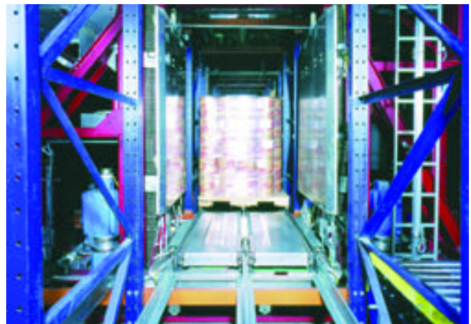
3. Order picking is serviced by fully automatic selective vehicles.
